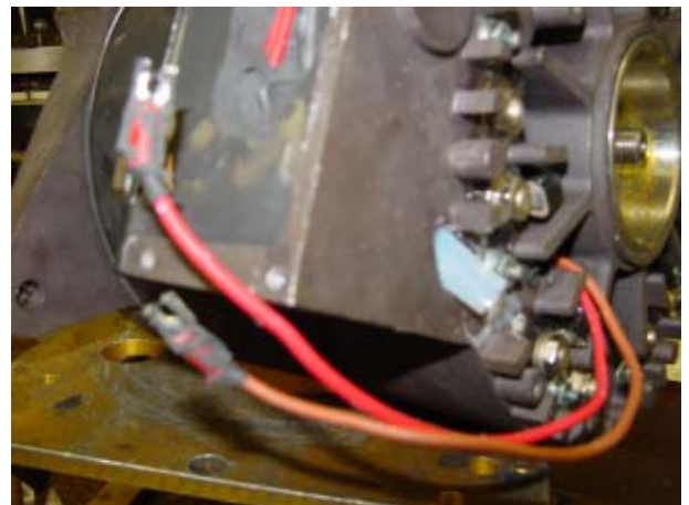
Figure 2 – Field Coil Leads Removed from Control Unit
